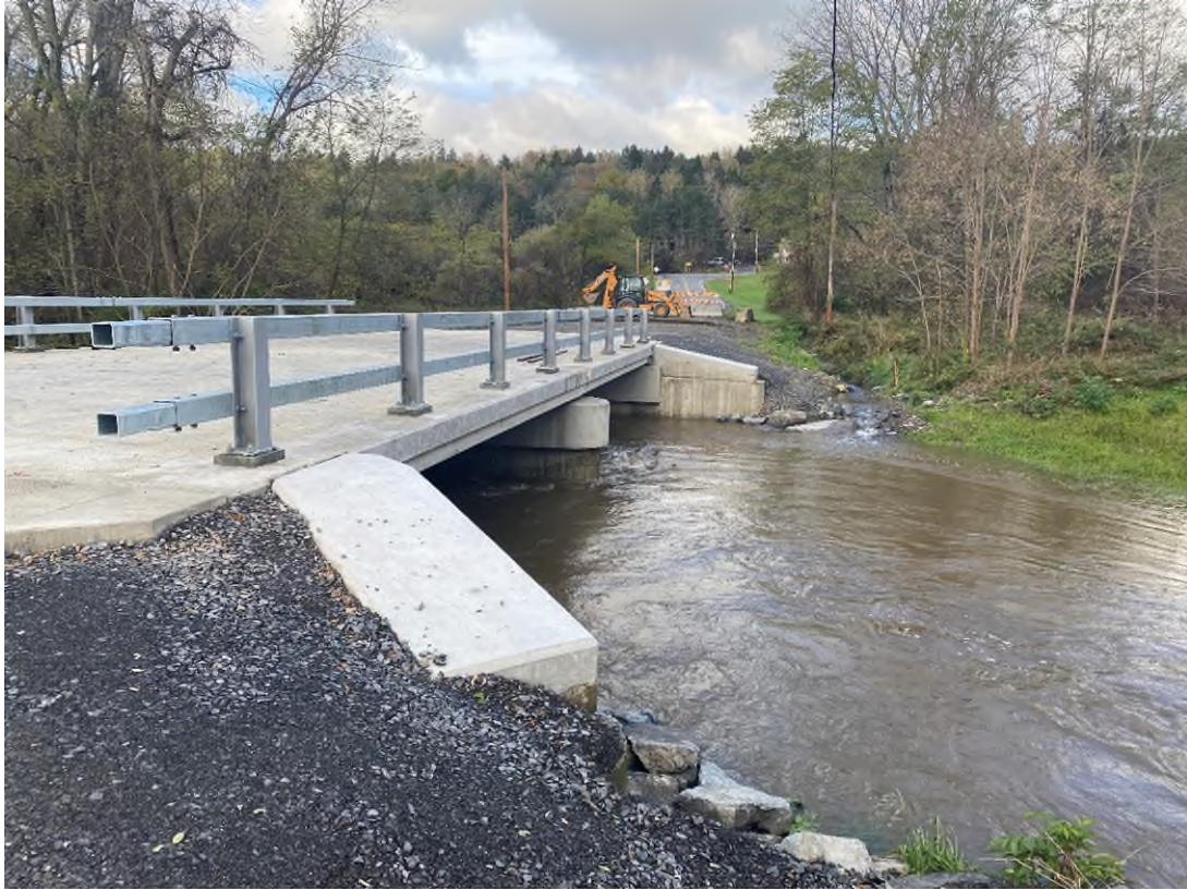
East Sherman Hollow – High water after storm event
