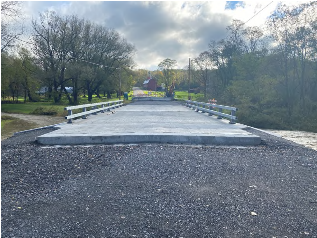
East Sherman Hollow – New deck and approach slabs, looking East, ready for HMA
